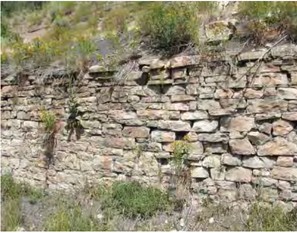
Rustic stone retaining wall reinforces the connection of the built environment with the landscape
